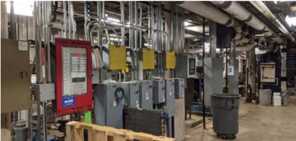
Images: Proximity issues of electrical gear and panels from mechanical, plumbing, and fire protection distribution in central plant.
